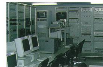
デジタル放送実験設備 Experimental equipment of digital broadcasting
