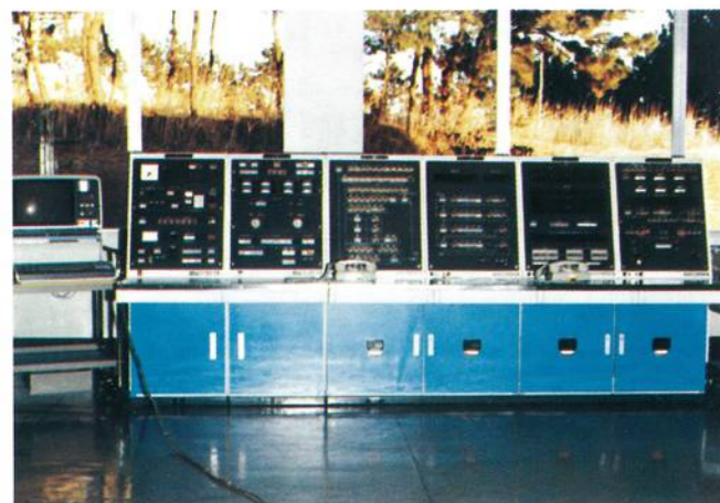
Satellite Control Panel, Kashima
