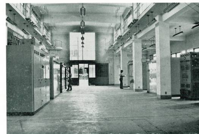
JJY Transmitter Room.
