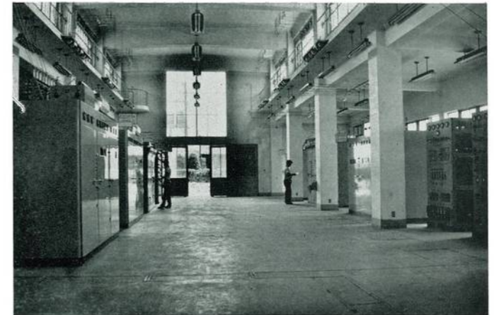
JJY Transmitter Room
