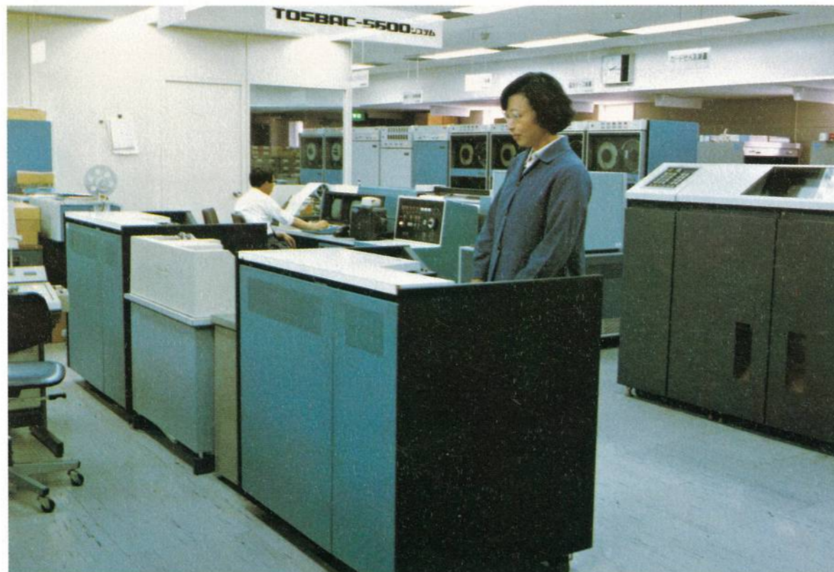
Main computer room
